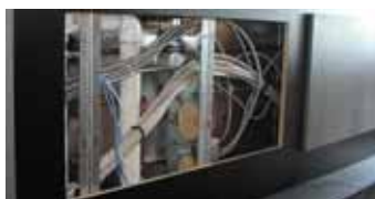
removable front panels expose the chase for repairs and modifications.
